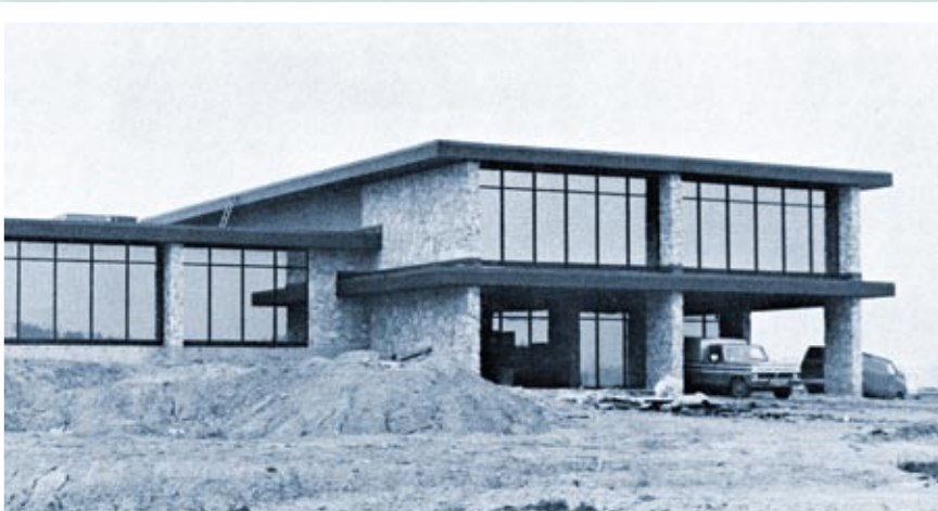
Ground was broken on the AFTMA Center, located in Arlington Heights, Ill., in 1977.
